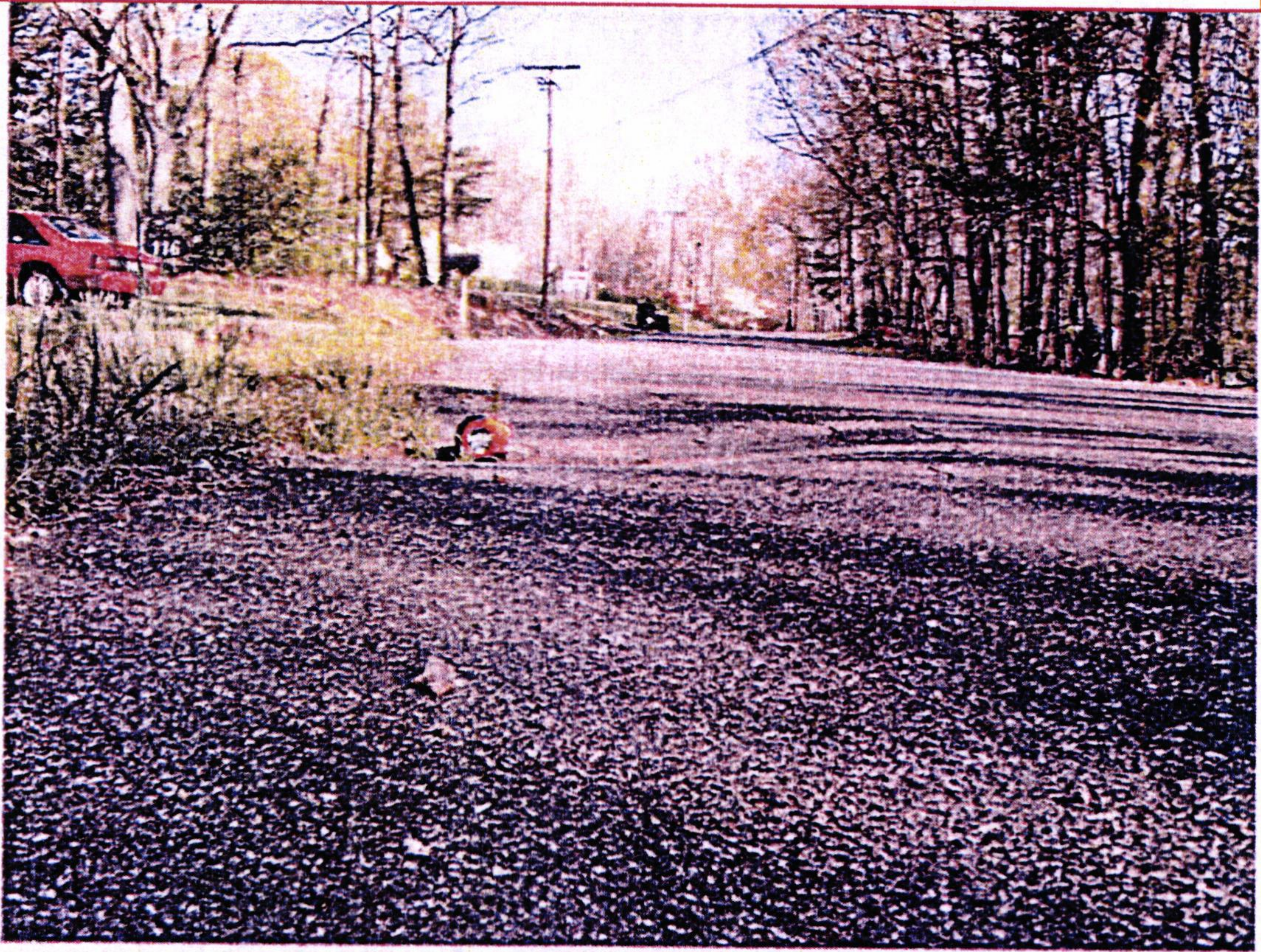
DEVELOPING POT HOLE ON 3 RD STREET SE
