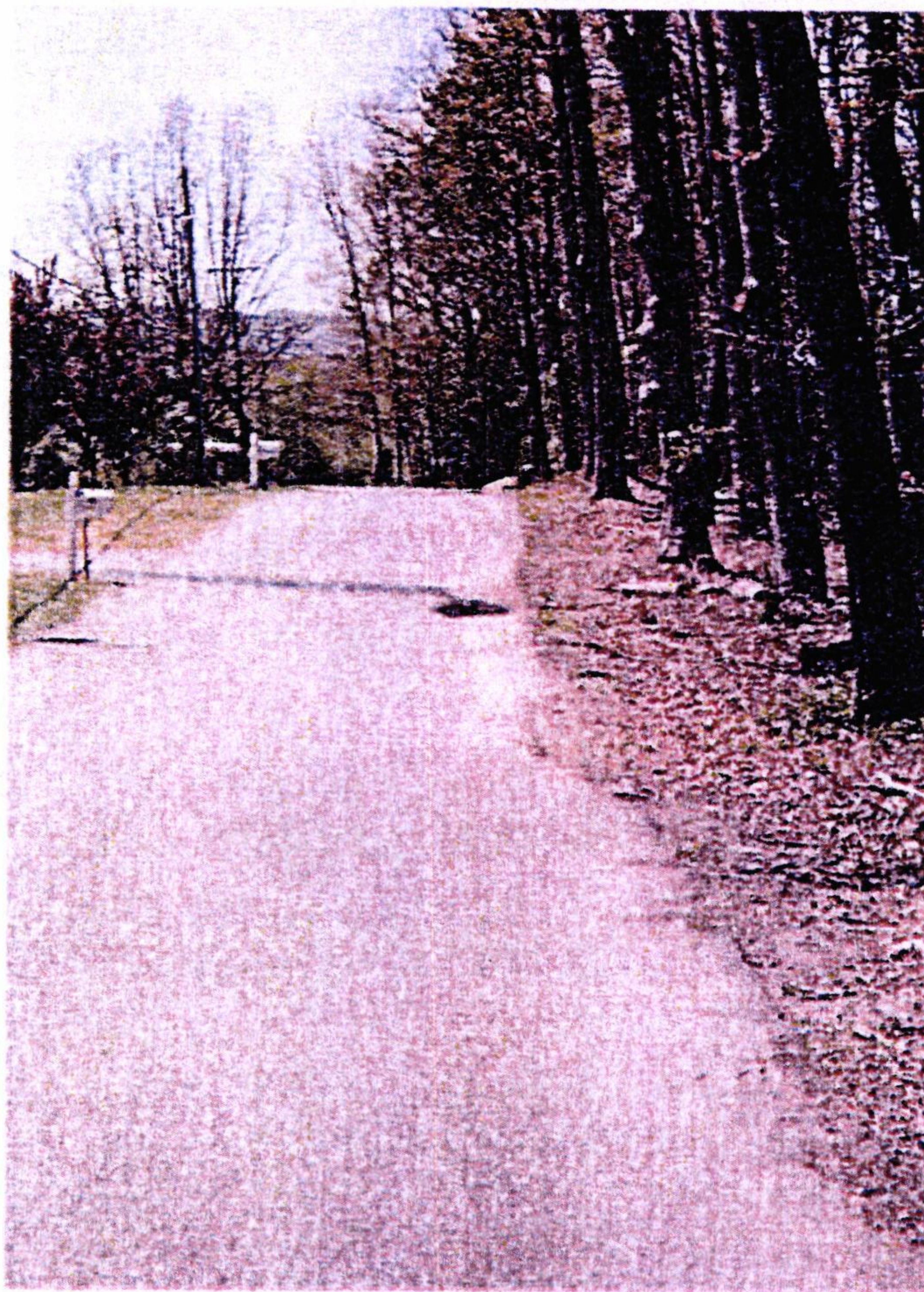
3 rd Avenue NW Shoulder Too High Blocking Runoff
