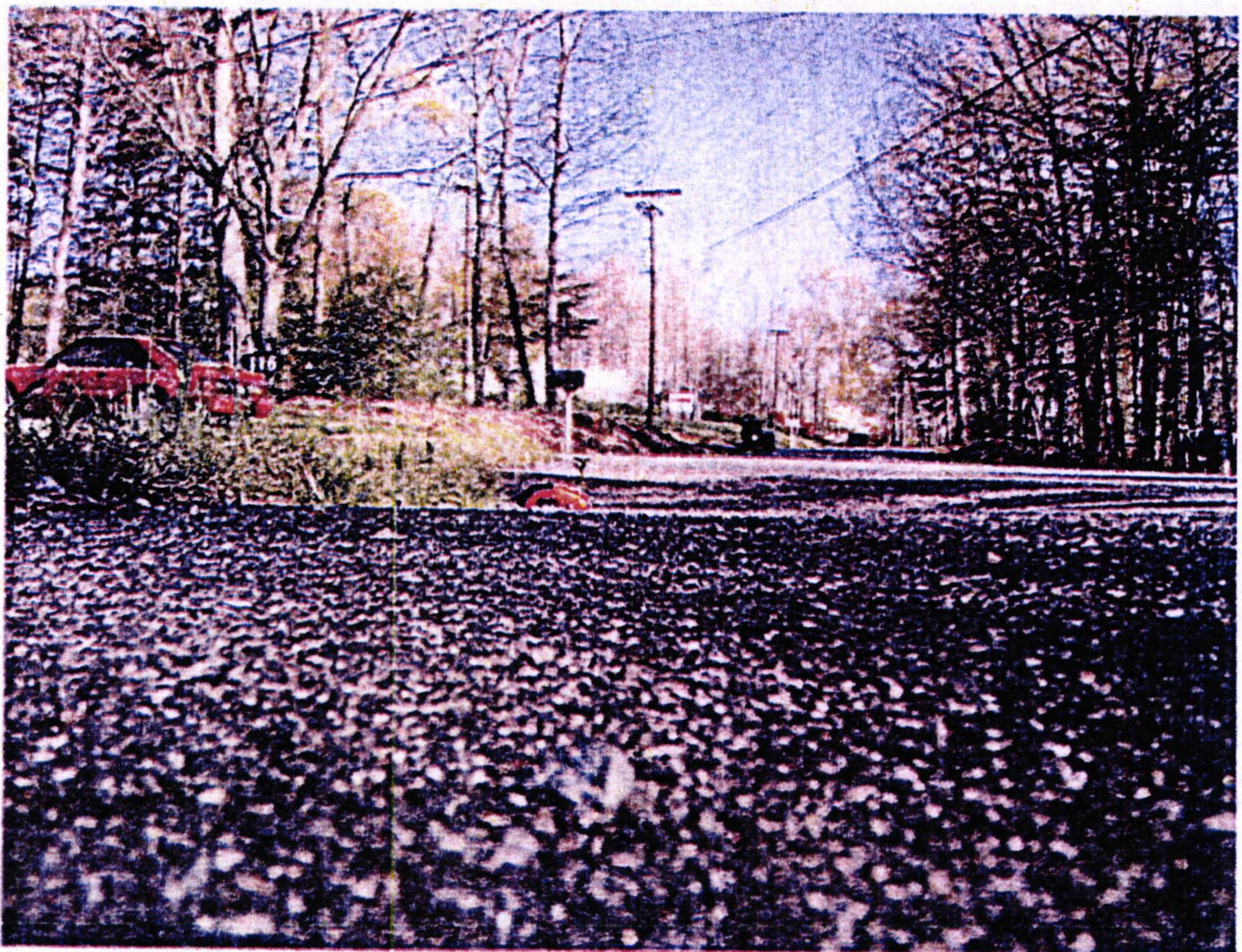
DEVELOPING POT HOLE ON 3 RD STREET SE (ABOUT 2" OF SETTLEMENT)
