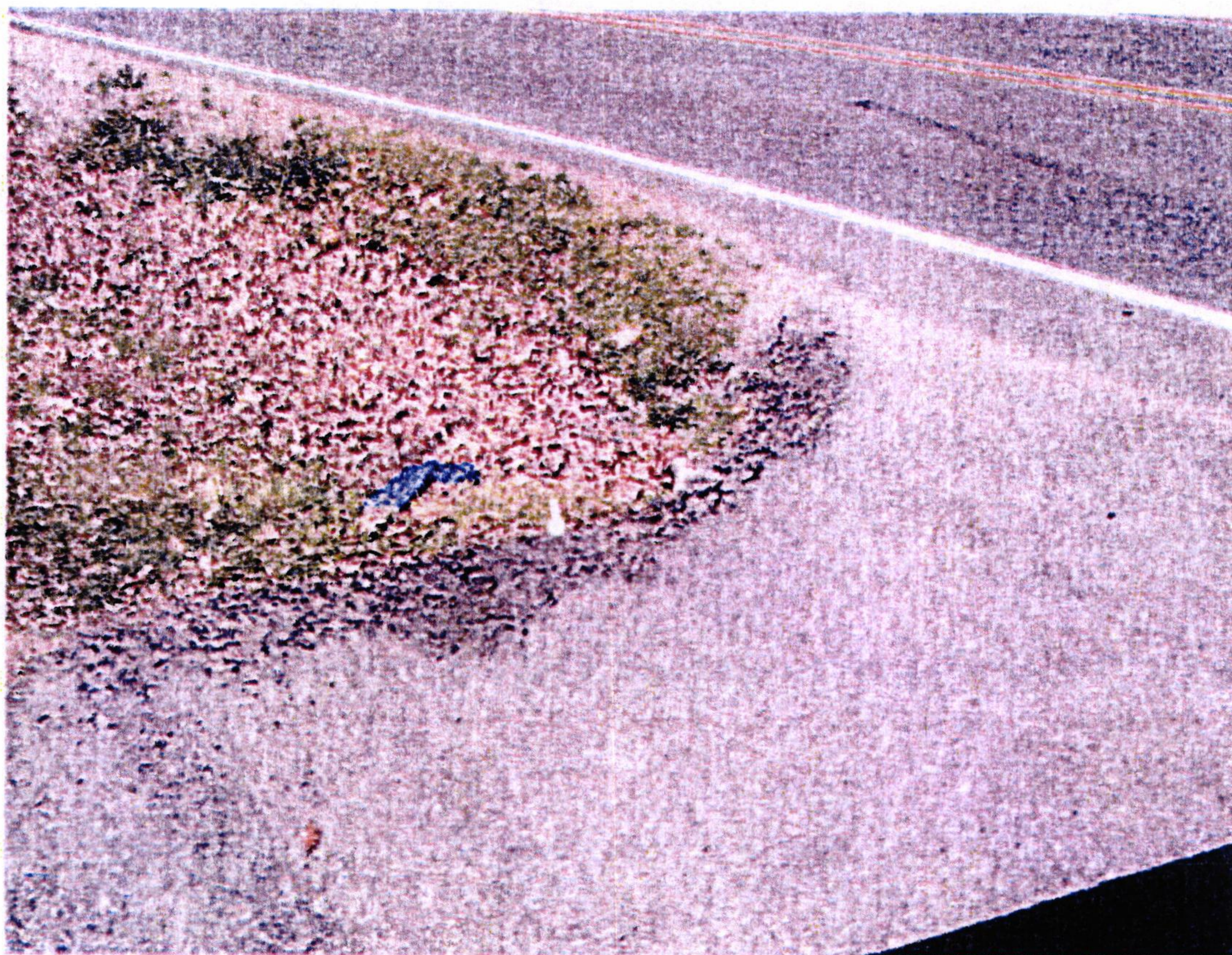
3 rd Avenue NW Entrance Pipe Needs to be Extended
