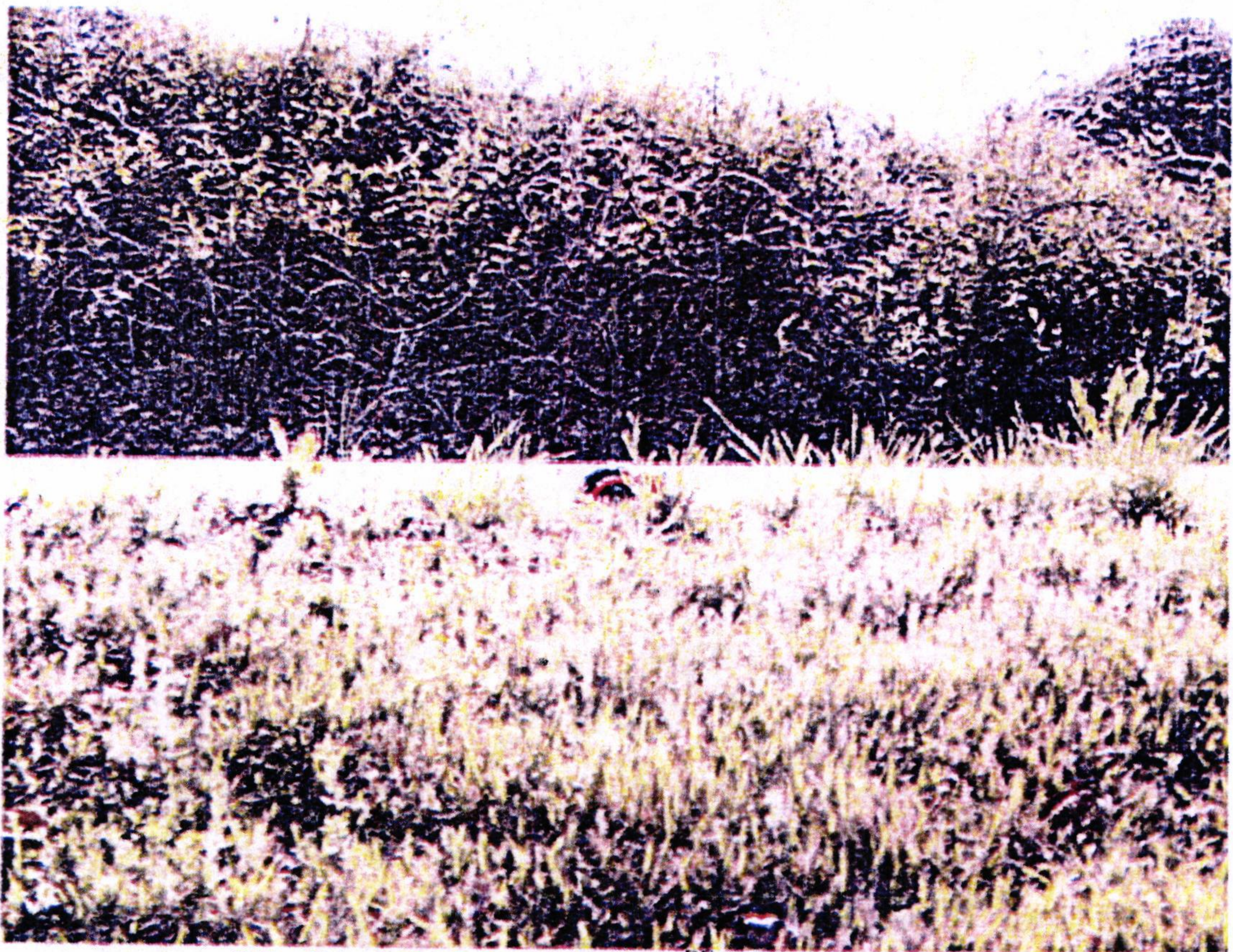
DRAINAGE PROBLEM ON 3 RD STREET SE EXT. GRASS SHOULDER SHOULD BE TRIMMED DOWN TO ALLOW RUNOFF TO EXIT ROADWAY (ABOUT 2")
