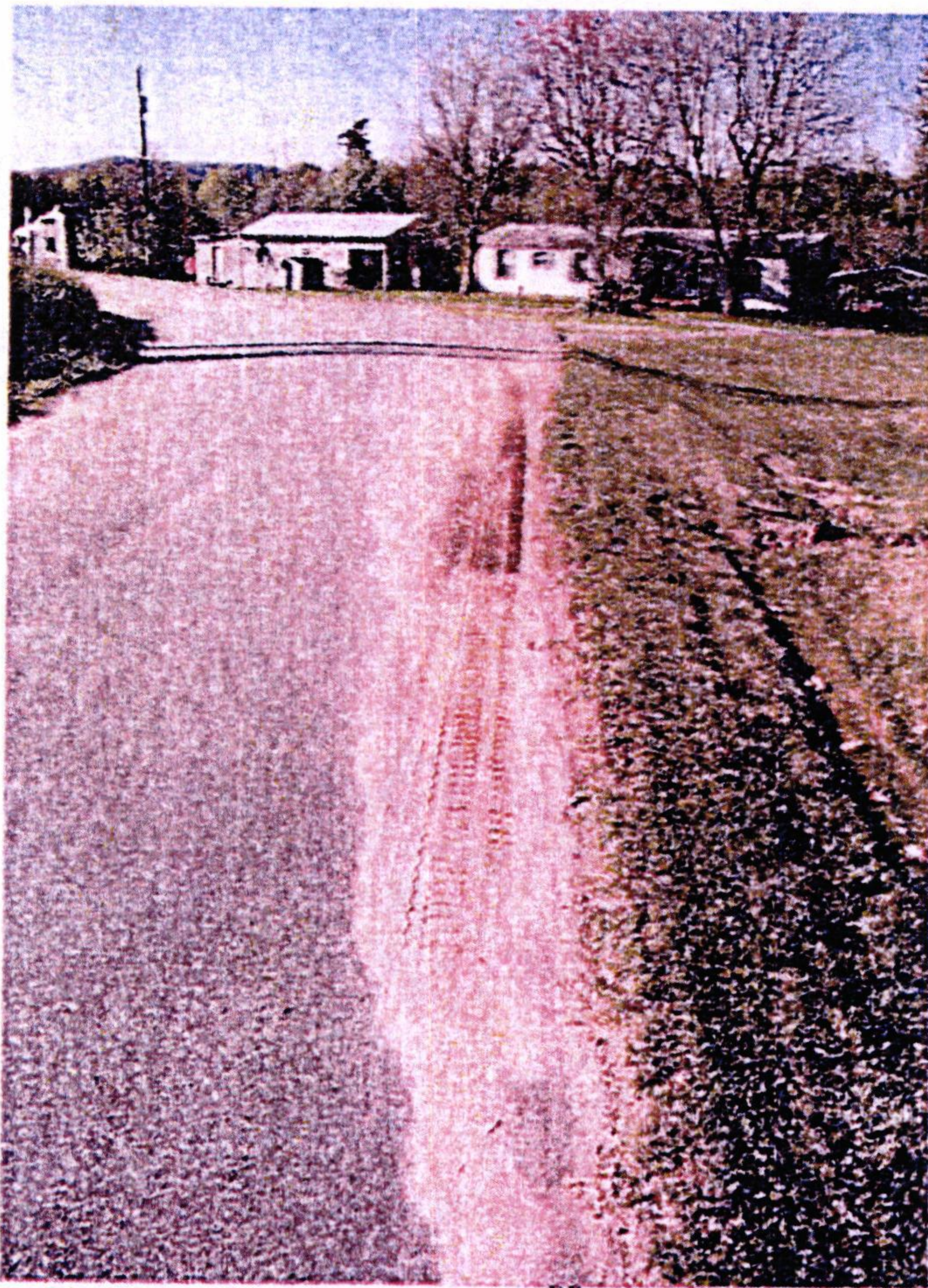
DRAINAGE PROBLEM ON 3 RD STREET SE EXT.
